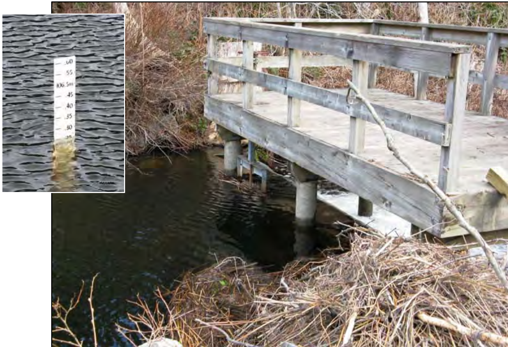
Photo 7. Outlet dam on Grafton lake and beaver dam debris removed by BIM staff. Inset shows water level of 105.20 m on that date. 25-Mar-09
