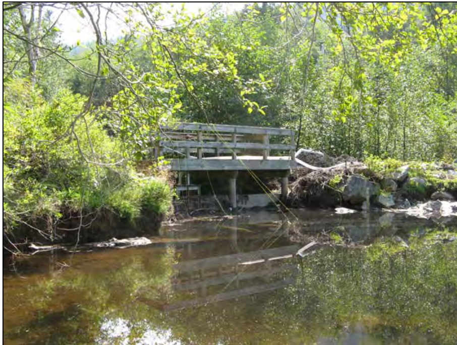
Photo 9. Grafton lake outlet dam during summer draw-down. Ropes attach to outlet pipes installed through under drain to overcome damming by beavers and ensure compliance with water release requirements to Terminal Creek. 19-Aug-09
